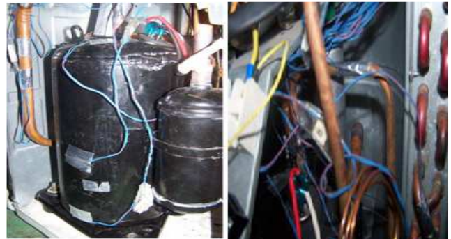
Figure 3. Compressor with thermocouples.
